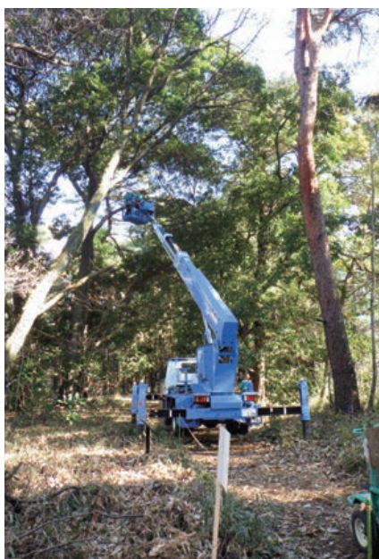
Photograph 7 Securing the safety of the tour route using aerial work platform vehicles Hanging and dead branches are removed.
